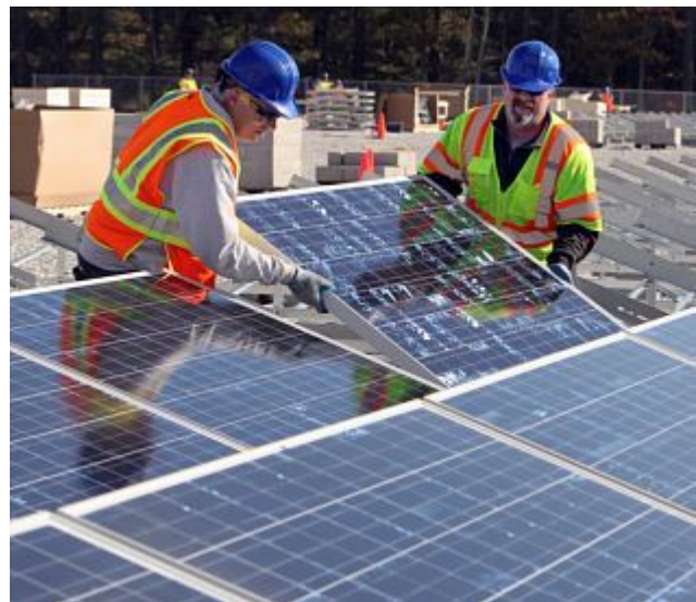
READY TO SHINE: Electricians Frank Perotta, left, and Tony DeSantis install solar panels at the new Westford Solar Park, set up by private developers.
