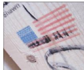
An American flag stamped on a pine 2-by-4 shows that the wood framing used at two new buildings at Church Landing is American-made. BRENDA CHARPENTIER
